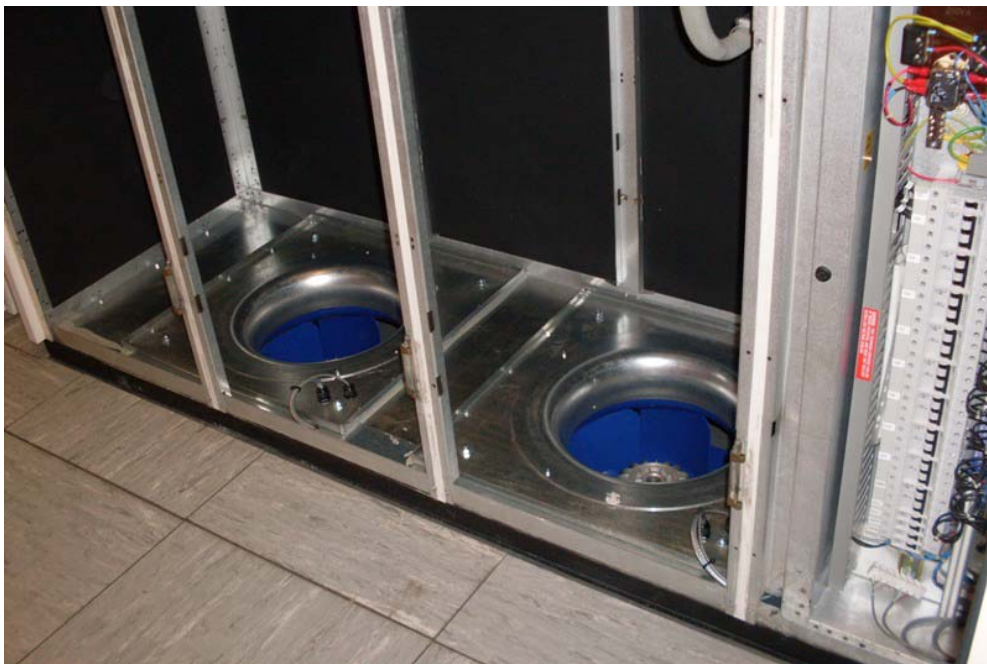
The new system has been equipped with high efficiency, backward curved EC fans
