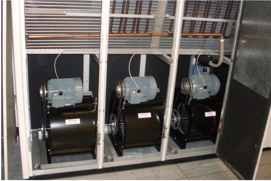
The old system at O2 Runcorn used forward curved fans
